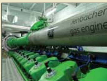
GE's innovative Jenbacher cogeneration technology is being used at Ploiesti.
